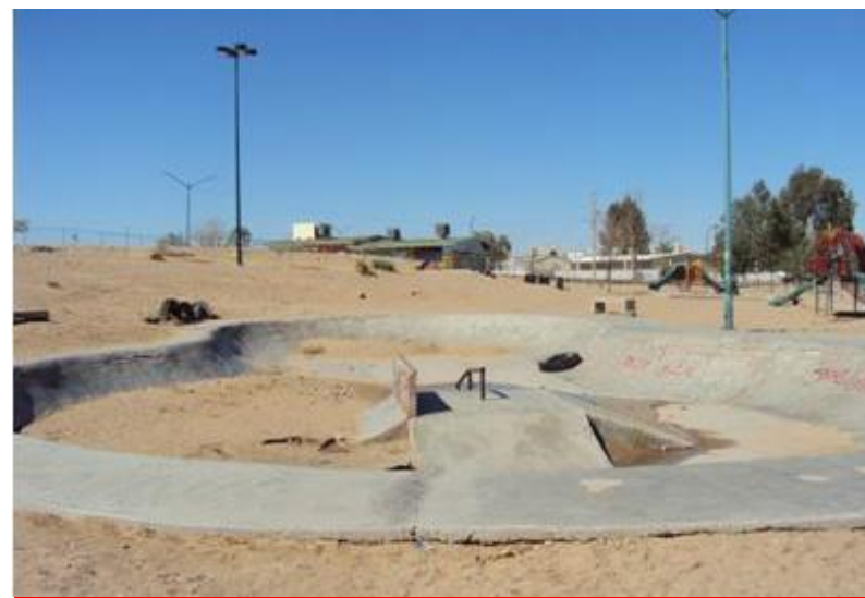
In state of neglect
